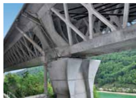
KKS corrosion protection for the supports of the "Sylans viaduct" in France
